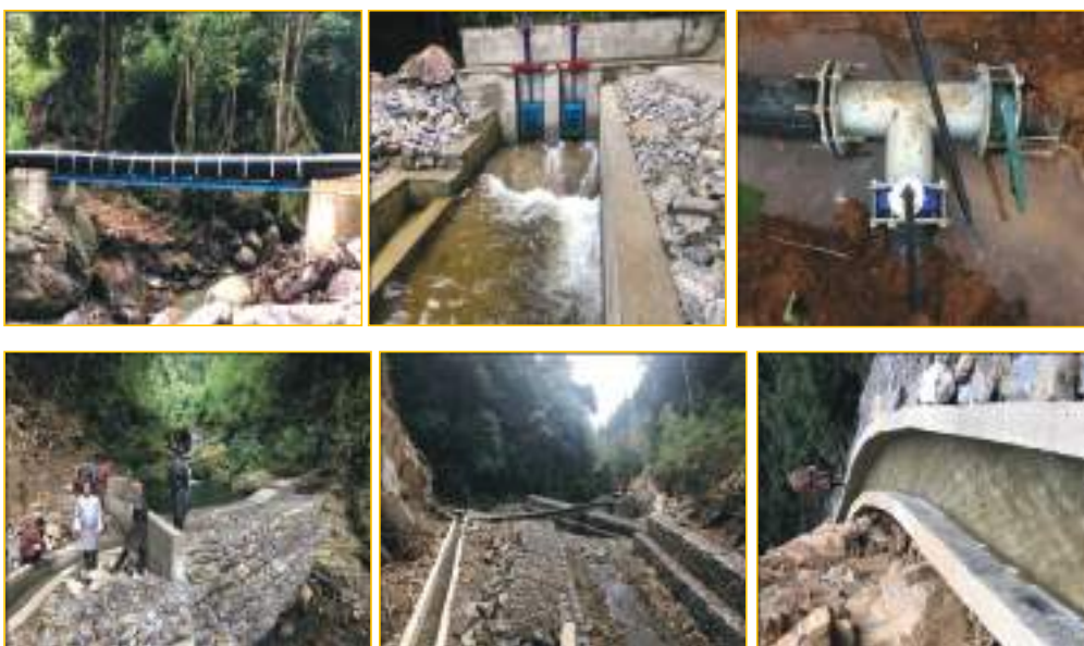
Figure 32 Structures at Phendey Yuwa, Talo, Punakha (top row) & Jhatey, Sergitahng, Tsirang (bottom row)
