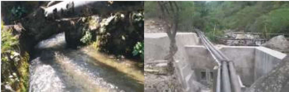
Figure 29 Initial Intake structure (left) and present intake structure (right) at Baychhu (Wangdue)
