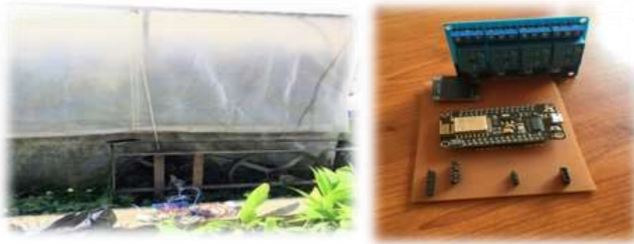
Figure 27. Automated Roll up motor for ventilation (L) & Printed Circuit Board (R)
